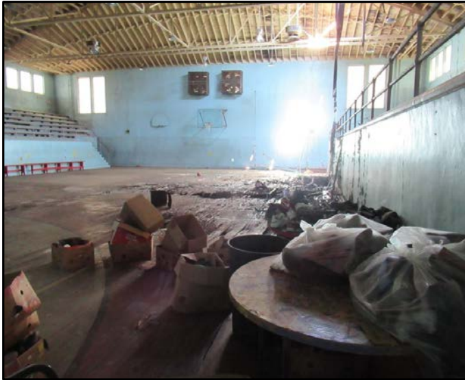
looking toward hole in gym floor
