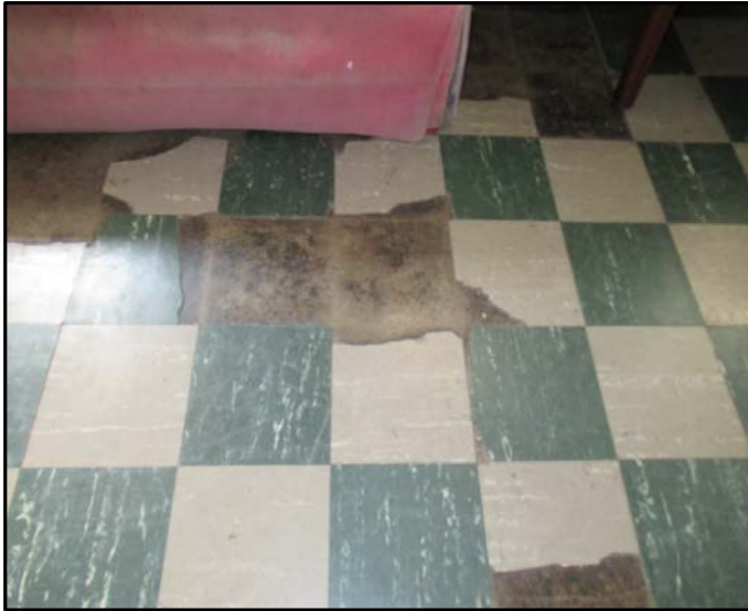
Broken, missing tiles, classroom
