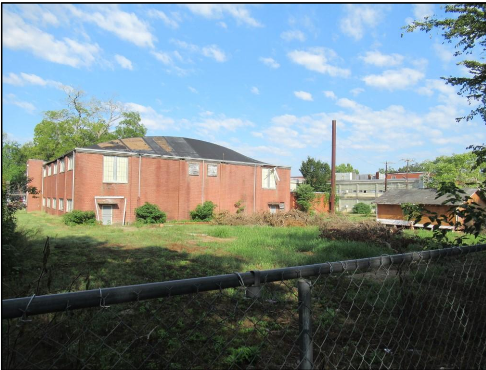
Damaged membrane roof of Gym
