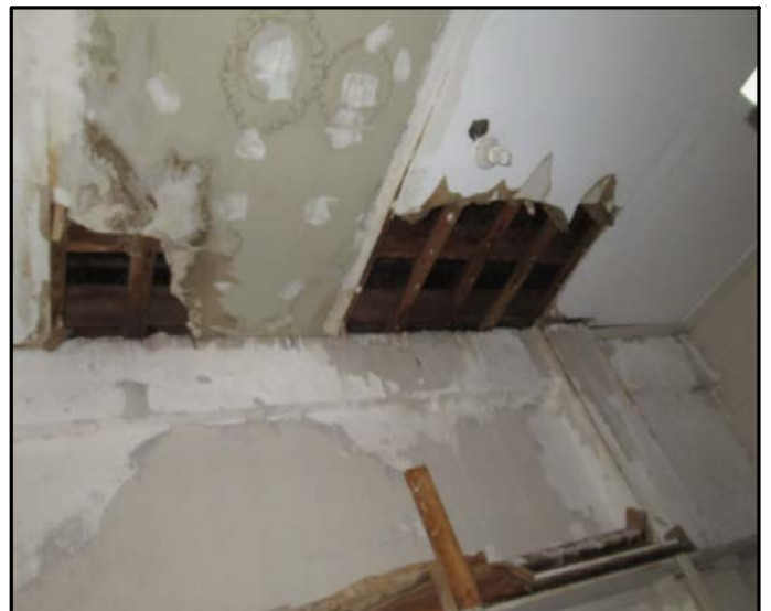
ceiling damaged upstairs.
