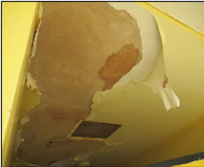
paint peeling, damaged plaster
