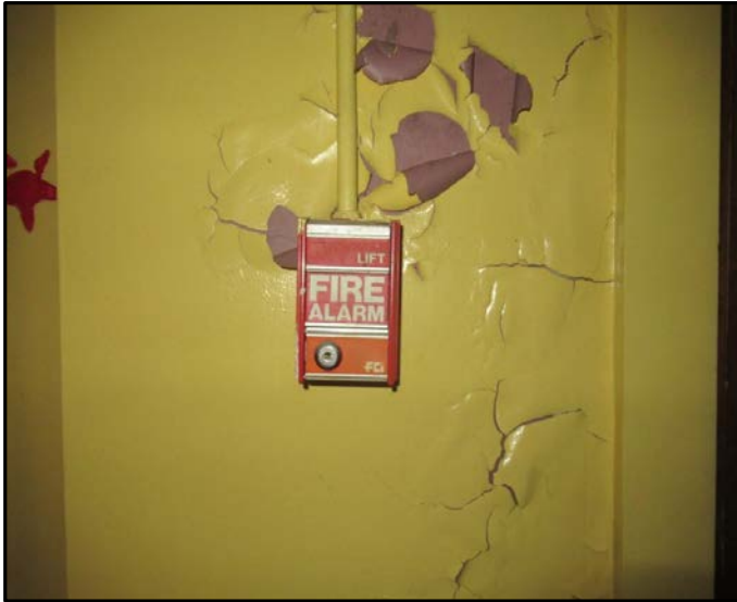
Peeling paint in hallway
