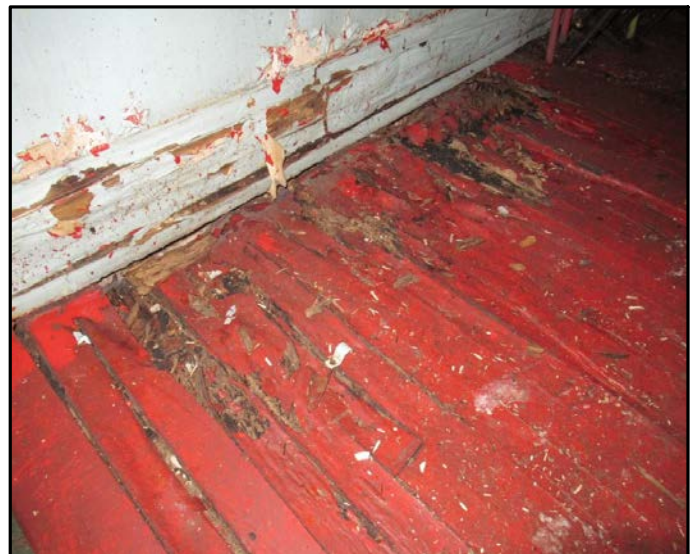
wet and rotted wood floor
