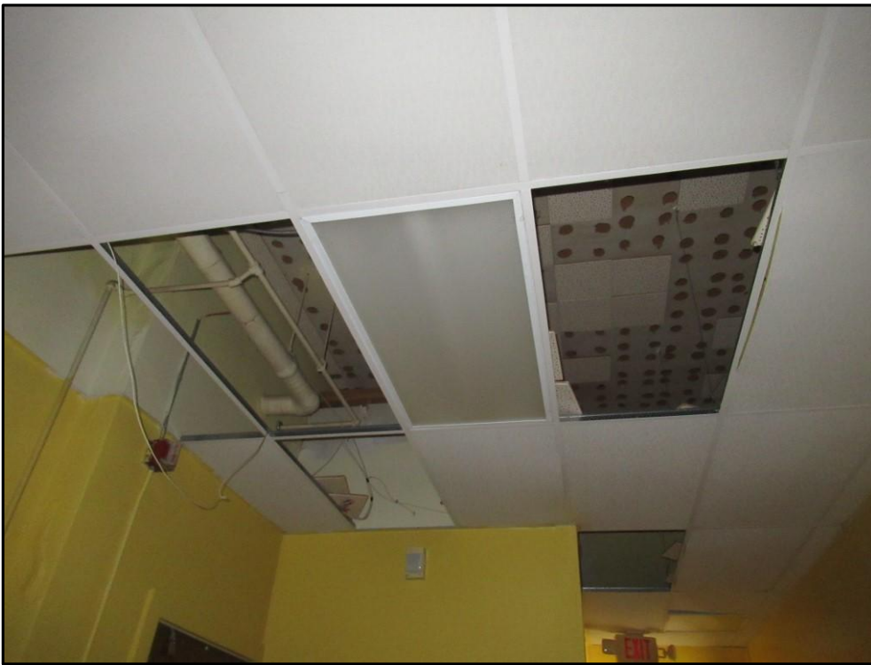
New tile falling down from leak
