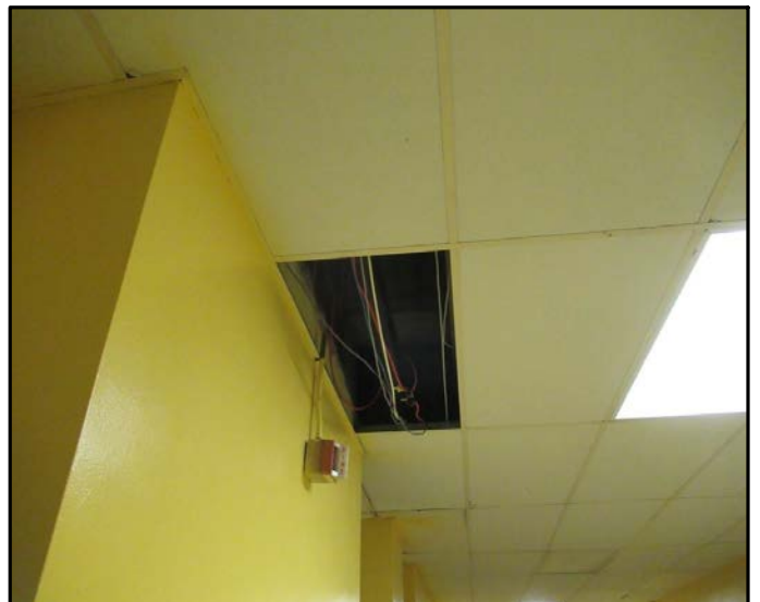
ceiling panel missing
