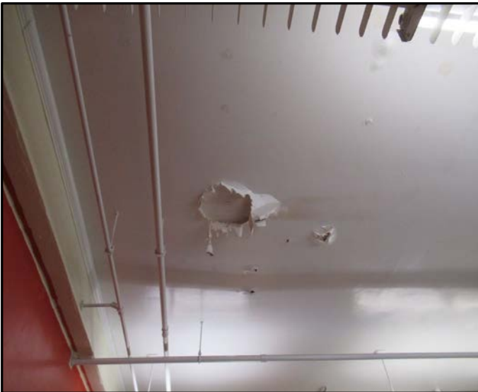
peeling paint on ceiling
