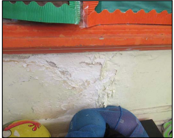
peeling paint, disintegrated plaster
