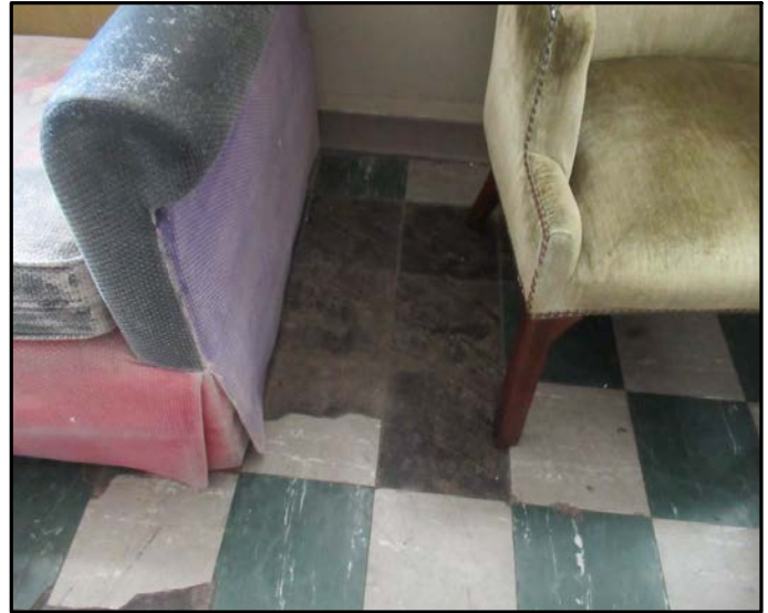
Broken, missing tiles
