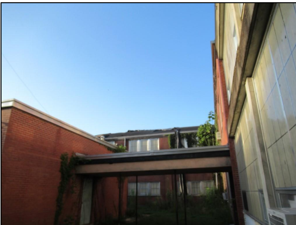
looking toward damaged roof on gym
