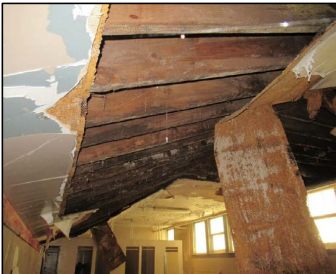
water damage to ceiling
