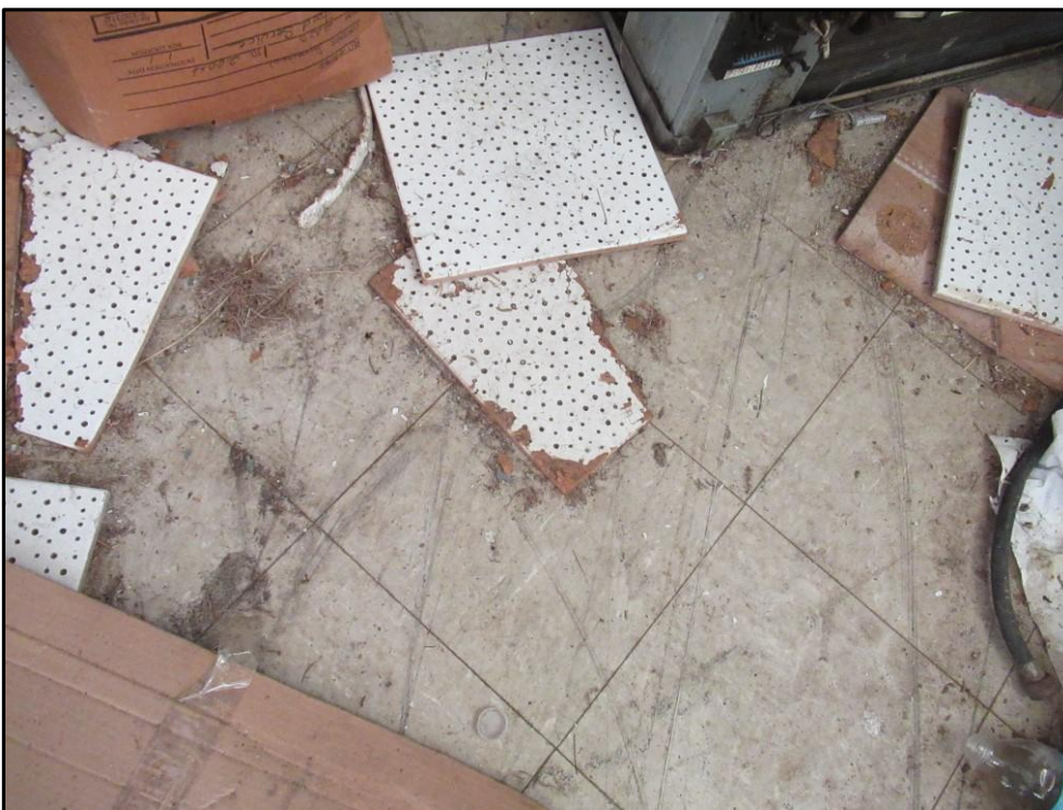
Tiles & flooring possible asbestos
