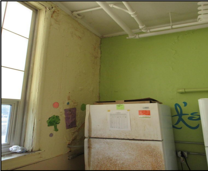
Damaged plaster from water
