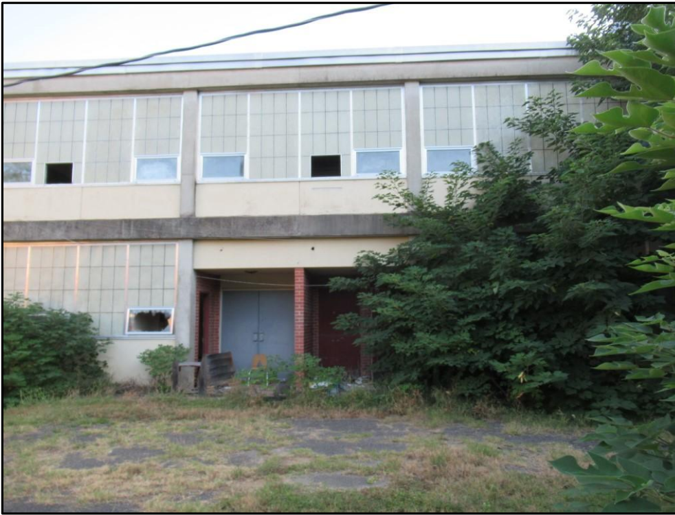
Missing glass & AC units
