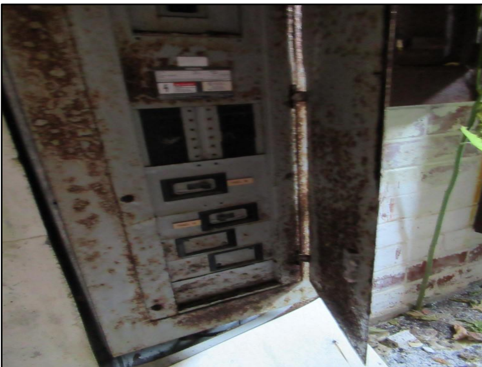
Electrical panel in boiler bldg
