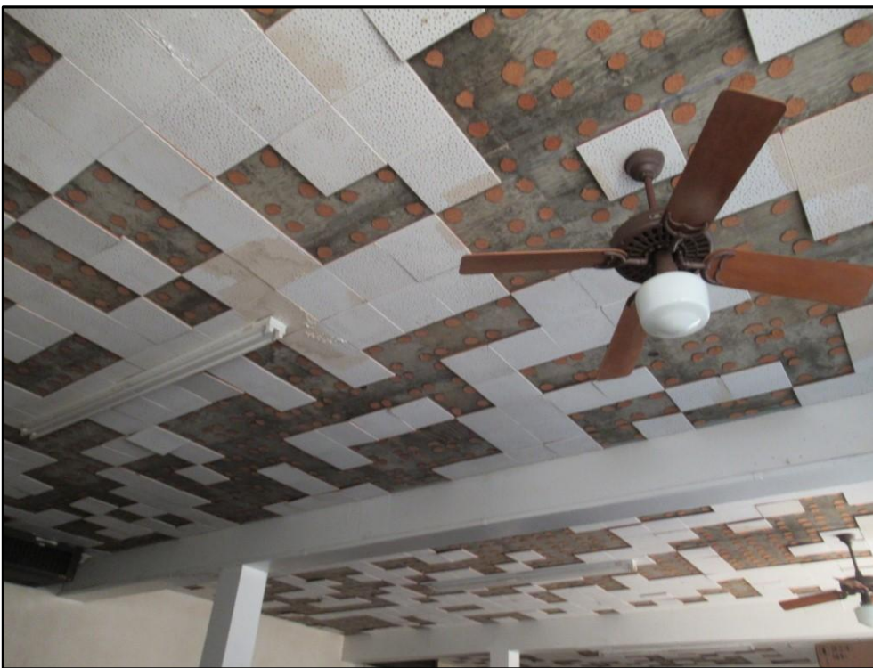
Tile falling off ceiling of cafeteria
