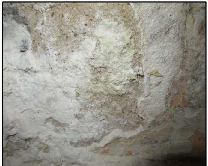
Plaster disintegrated plaster
