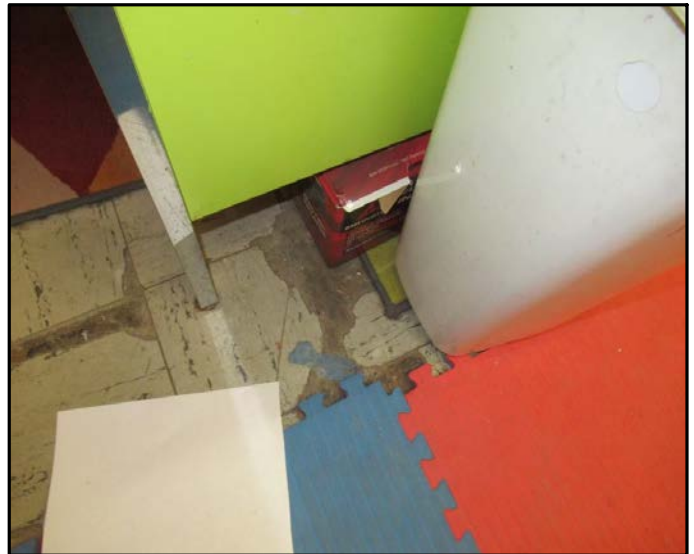
Broken floor tiles
